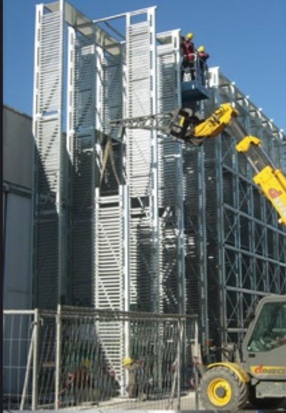
EXTERNAL UNICO installation of an Unico outside the factory
